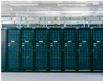
DATA STORAGE & SERVER FARMS
